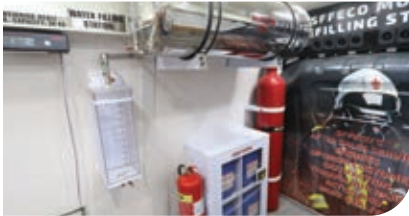
Foam / Water Filling Station
