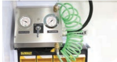
Extinguisher Pressurizing Unit
