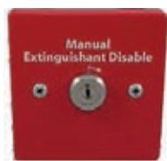
Manual Disabling Switch
